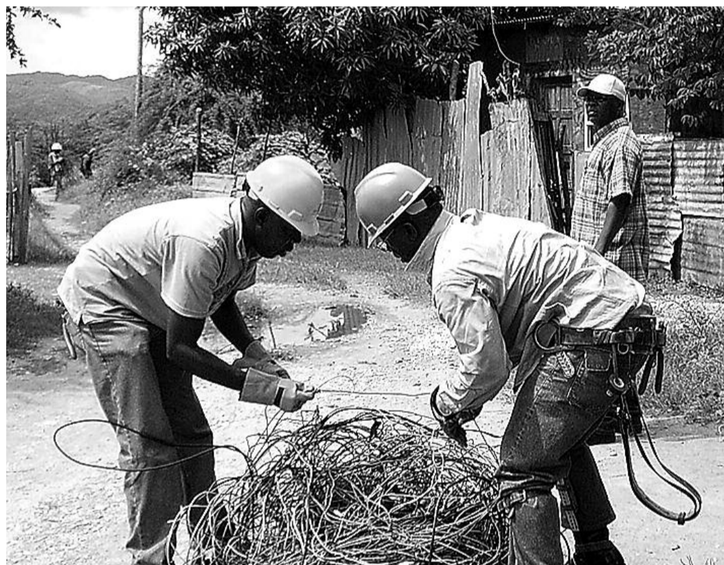
JPS workers gather illegally connected wires, which were removed in a raid in a St. Catherine community.
